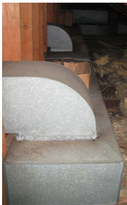
Miscellaneous duct conditions.
