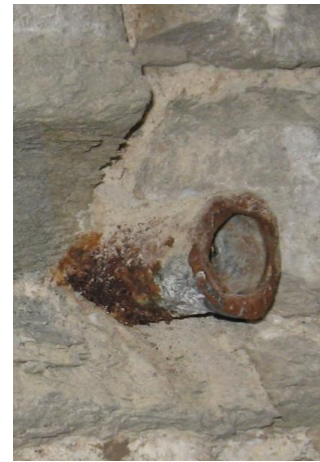
Electrical Distribution Panel and Circuitry - Detail view to existing non-code complying panel and meter [LEFT], and abandoned conduit in ground level west wall [ABOVE].
