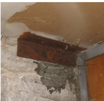
Detail images depicting ca. 1970 steel clip angles at first level floor framing.
