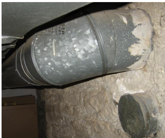
Miscellaneous duct conditions.
