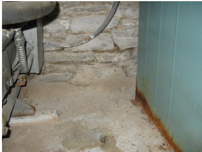
Detail images depicting the condition of stone masonry foundation system, including washed out mortar joints and effloresced stone units in mechanical room west wall [LEFT and ABOVE RIGHT]. Note the quantity of detritus on the floor, as well as the rusted base of HVAC equipment.
