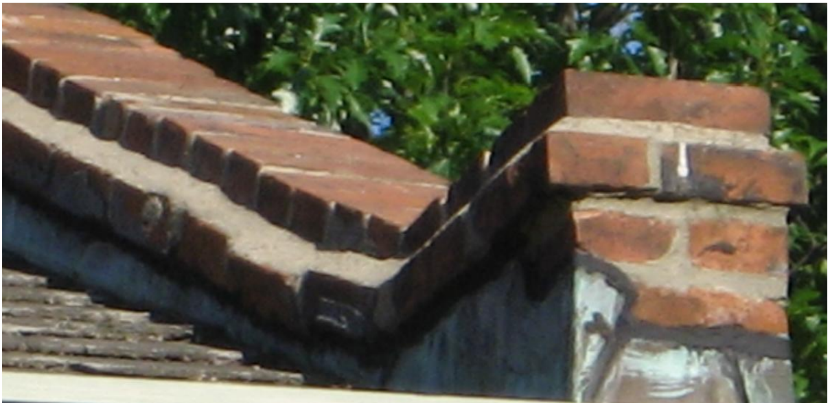
Exterior Clay Brick Masonry - Detail image depicts the design of masonry parapet cap [ABOVE] at Hanley House NE corner. Sheet metal step flashing engages back-side and end of parapet, with mortar wash applied from row-lock at top of parapet to first corbeled course. The undulating appearance of clay brick at the parapets suggests that they may have been repaired before.
