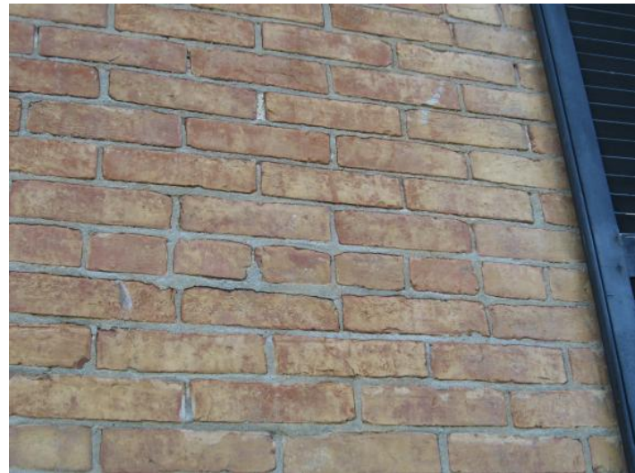
Note that south facing exterior clay brick masonry demonstrates a large variation in conditions - while some areas of wall are serviceable, there are several key faults which suggest movement in the multi-wythe brick masonry walls, with significant cracking of mortar joints and brick units.
