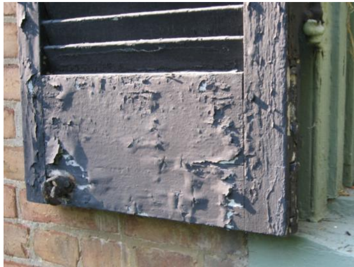
Detail image [LEFT] depicts the mortise-and-tenon construction method used to assemble original wood shutters at Hanley House - note desiccated and cracked condition of stile (vertical member), and off-set surfaces of the tenons as they appear at the left side of the stile.
