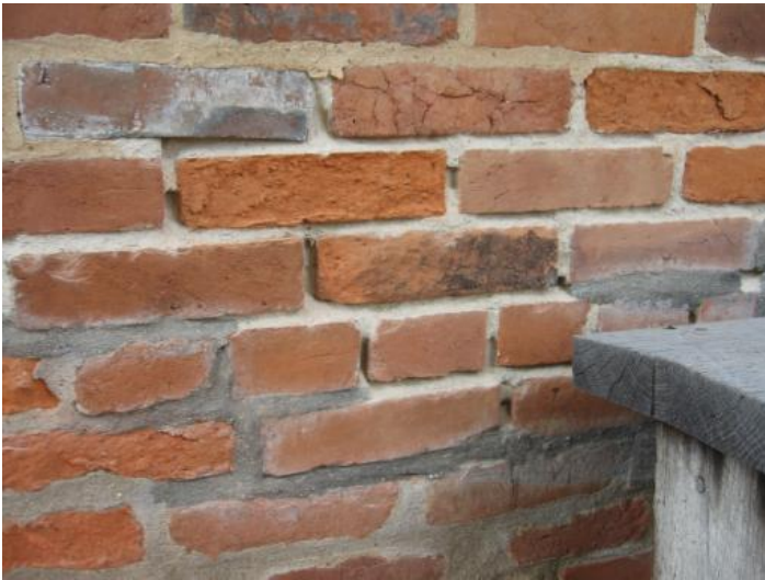
Detail at Typical Deteriorated Clay Masonry [TOP LEFT]
