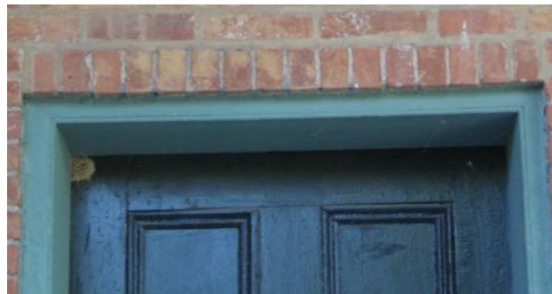
Detail images show typical wood exterior door design, including wood casing, trim and relationship to exterior clay brick masonry [ABOVE and LEFT].
