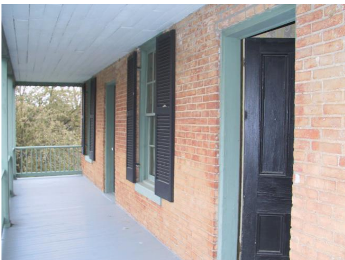
View to north at west porch second level [ABOVE] View to main entry at east elevation [RIGHT]
