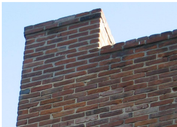
Detail images depict existing condition of clay brick masonry repaired ca. 1970 or after at SW chimney high points [ABOVE], and ceiling and beam pocket for roof at west porch second level [LEFT]. Note the contrasting color of mortar, and the relative depth of repaired joints.
