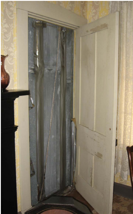
View to Typical Interior Duct Chase
