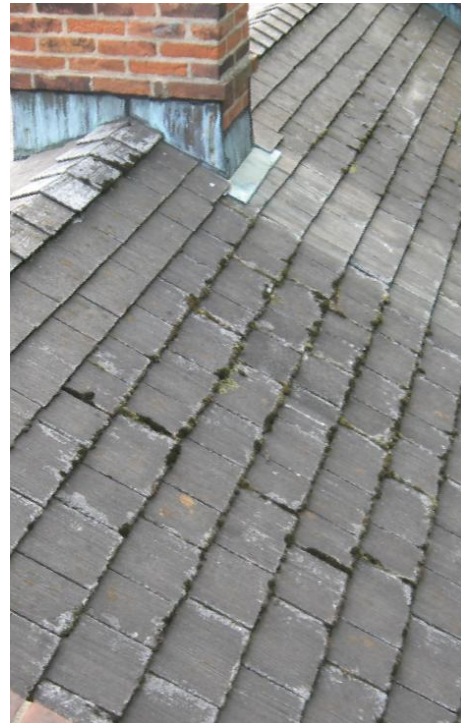
Detail at Typical Deteriorated Cement Tile Finish Roofing System [TOP RIGHT]
