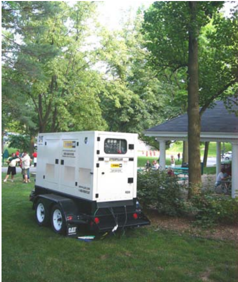
SHAW PARK , Electrical upgrades will include additional power pedestals to reduce supplemental equipment needs.
